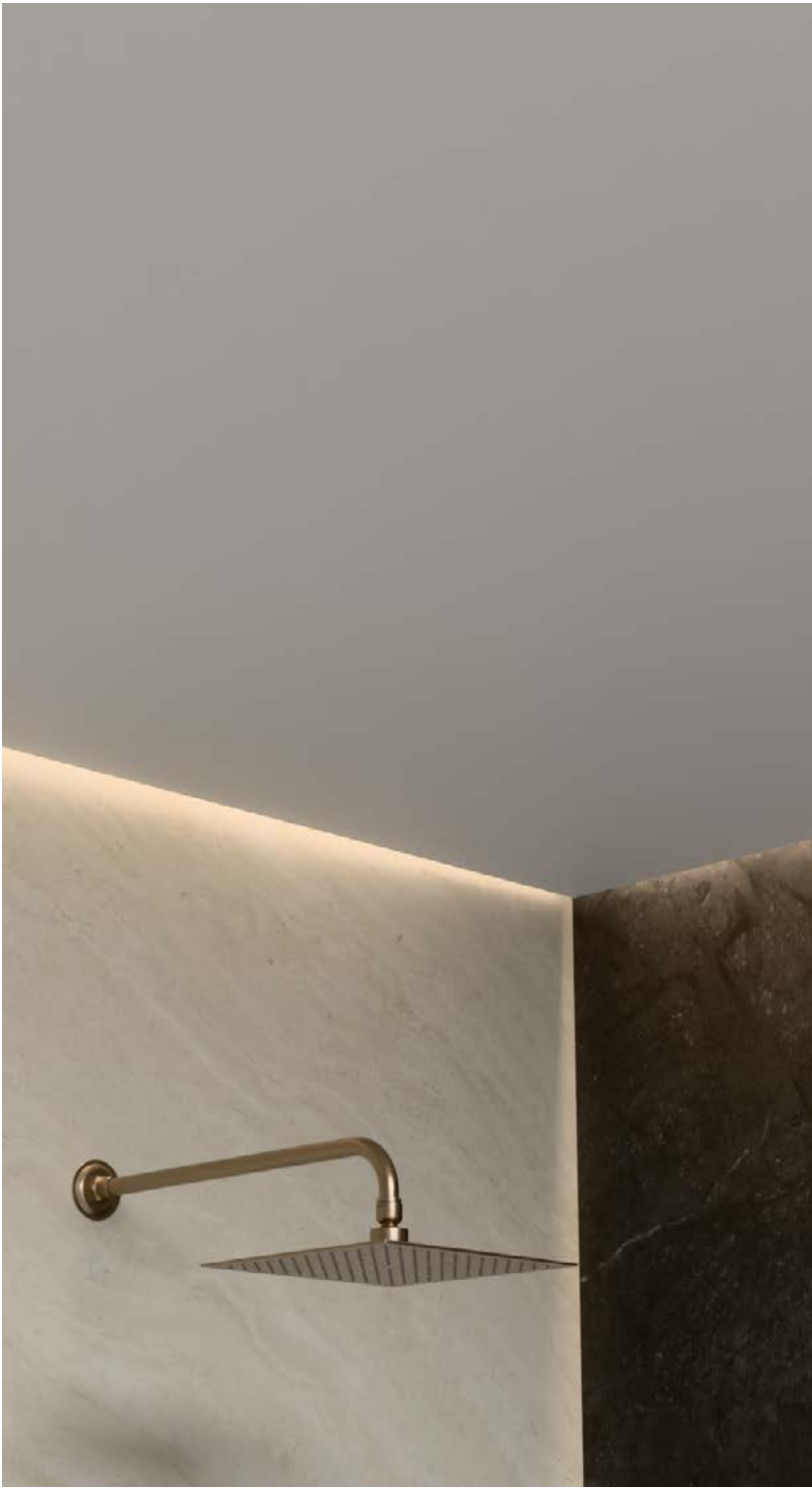
Wall Mounted showers.
